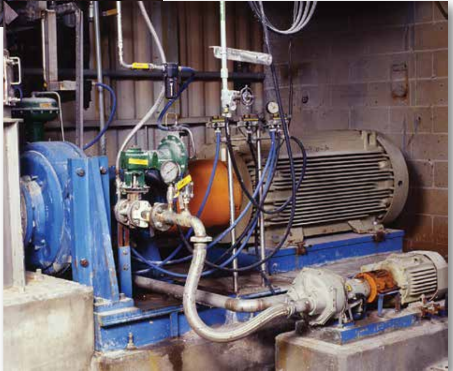
Bleached pulp from final wash stage being pumped to HD storage.
