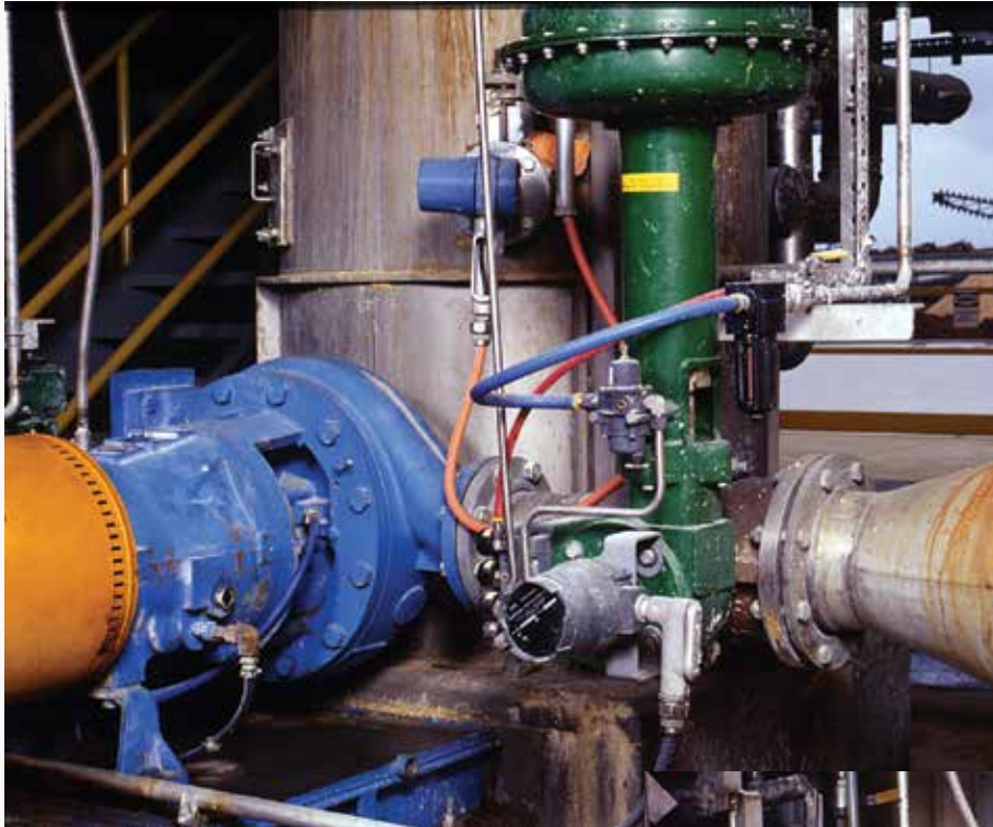
Caustic stage pumping from washer operating at 1200 TPD at 12% consistency. One of seven units in complete bleach line.
